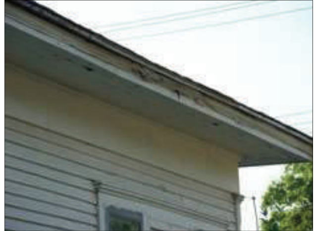
The soffit and fascia on this single-family home is rotting.
