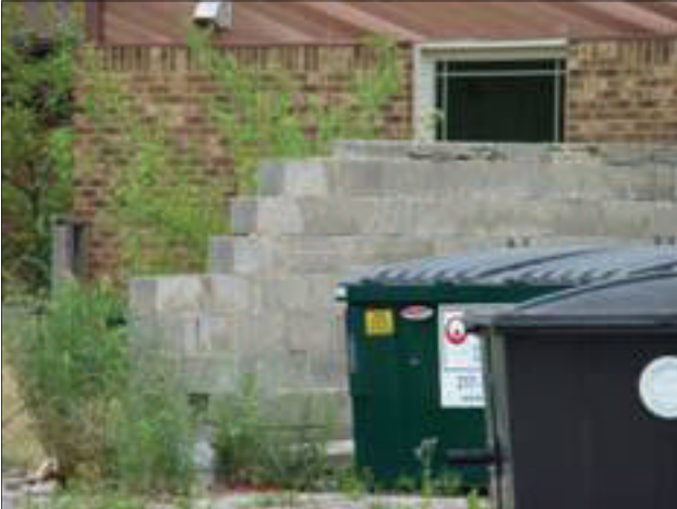
The dumpster enclosure wall is missing sections of cinder blocks and the gate is missing.
