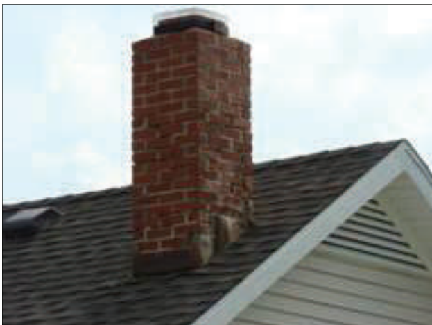
The chimney on the residential conversion shown above is in need of tuck-pointing and new flashing.
