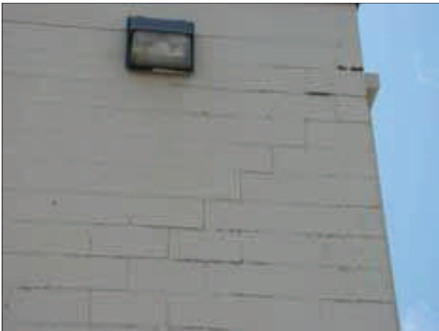
The side of the former retail building currently housing Illinois Employment & Training Center has severe step cracking.
