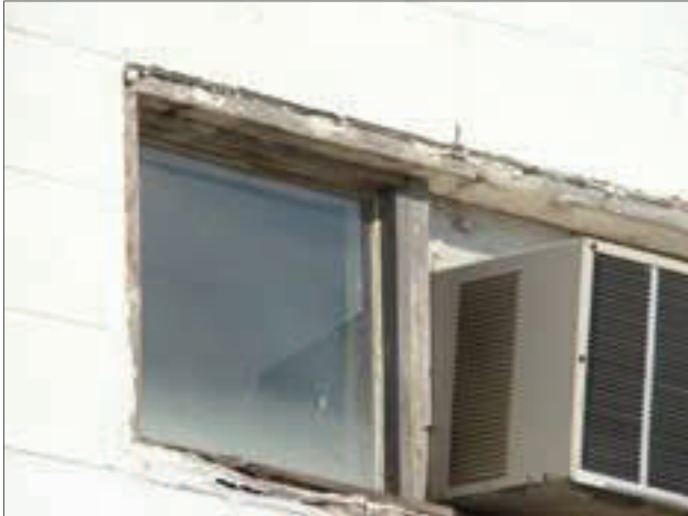
Window frames on the Monitor Sign Service building are rotting and in need of replacement.
