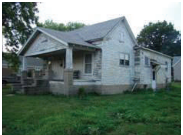
The wood siding on this home is also rotting.
