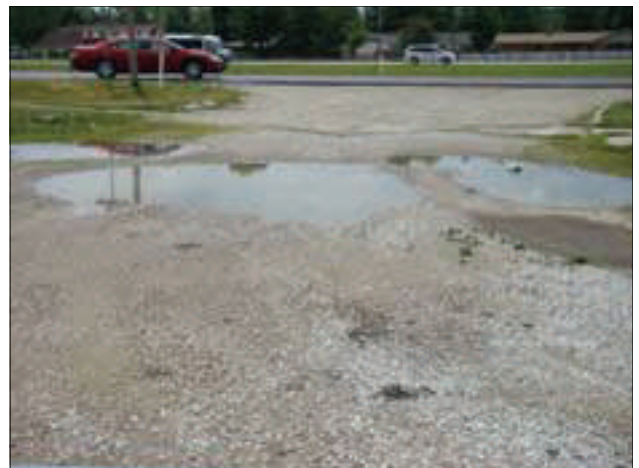
Potholes hold standing water in this dilapidated parking lot located along Broadway East.
