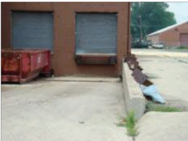
The railing along the loading dock behind CVS pharmacy has been knocked down and is lying in the alley.
