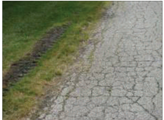
The rear drive to the medical office on Richmond Avenue is too narrow, resulting in vehicles rutting the adjacent lawn. Also not cracked, deteriorated pavement.
