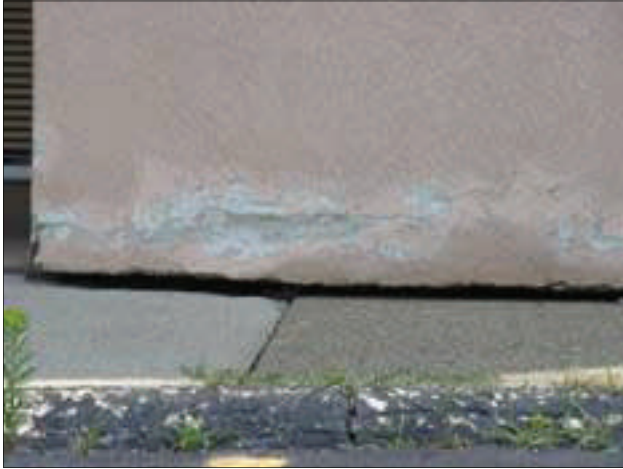
The exterior insulation finish system (EIFS) coating on the Ramada Inn is damaged in numerous places around the building.
