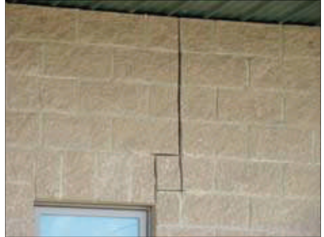
The side of this commercial structure along Shelby Avenue has several cracks such as this running down the wall.
