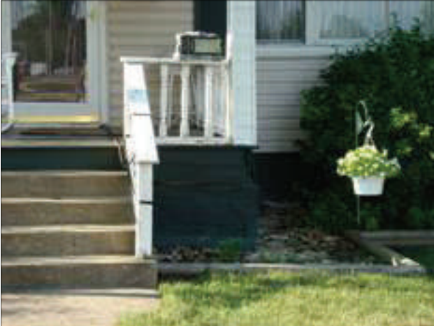
The porch on this single-unit dwelling is separating from the foundation.
