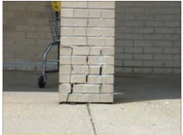
Columns on the front of this partially vacant former Wal-Mart building are cracking and bricks have become dislodged.
