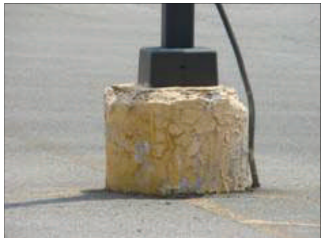
The lighting standards in the Big Lots parking lot are crumbling.
