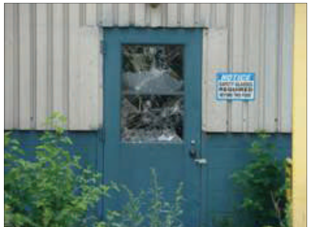
The glass in the rear door at Blaw Knox Ingersoll Rand has been shattered.
