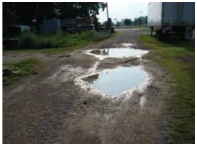
This deteriorated alley is typical of alleyway conditions in the Area, many of which are in need of resurfacing.
