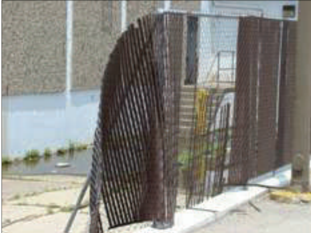
This fence near Big Lots is falling into the loading dock.
