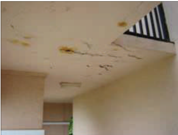
The ceiling at the Ramada Inn is cracking and peeling as a result of water damage.
