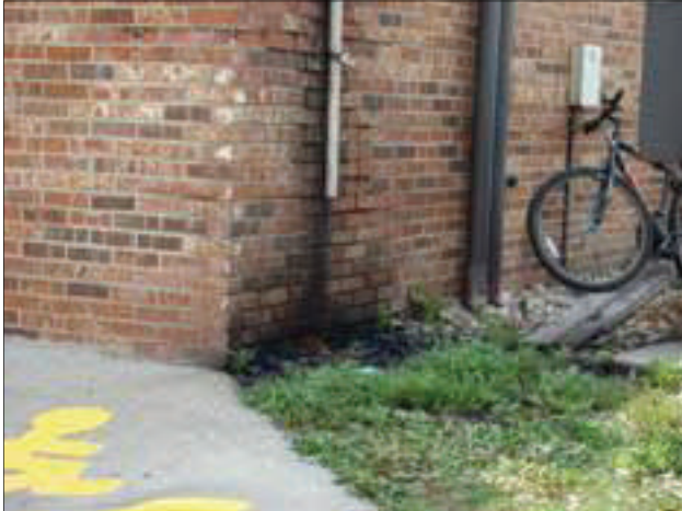
The rear of El Vaquero restaurant is missing sections of downspout resulting in mold growth on exterior walls.
