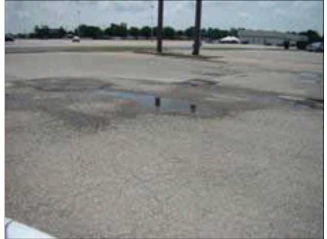
This parking lot serving the Dollar General is deteriorated and contains standing water.
