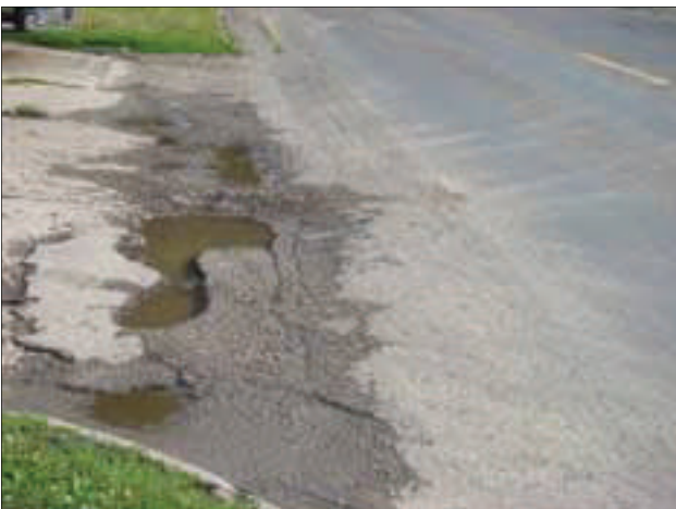
Many of the parking lot and driveway aprons throughout the Area are deteriorated and in need of repair.
