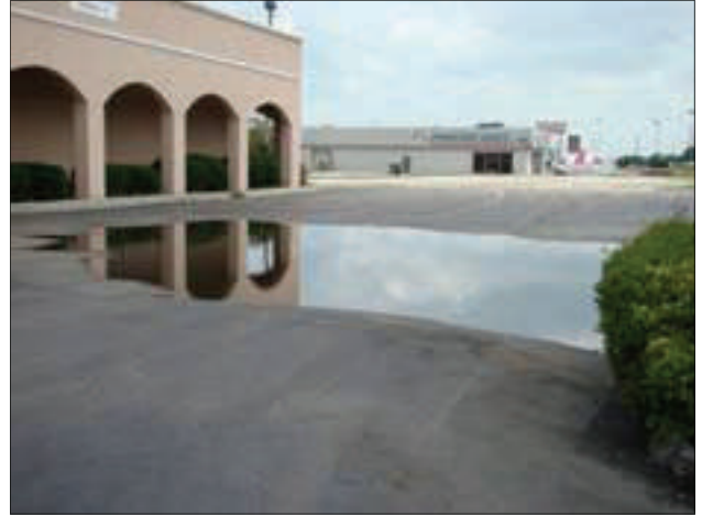
Large areas in the Ramada Inn parking lot hold standing water.
