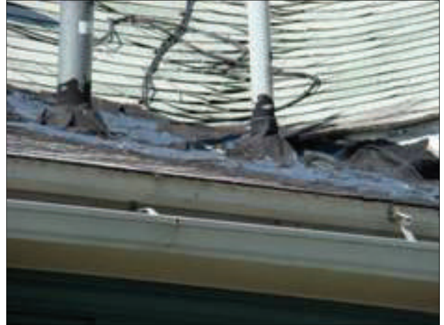
Roof repair is needed on this residential building on 11th Street.
