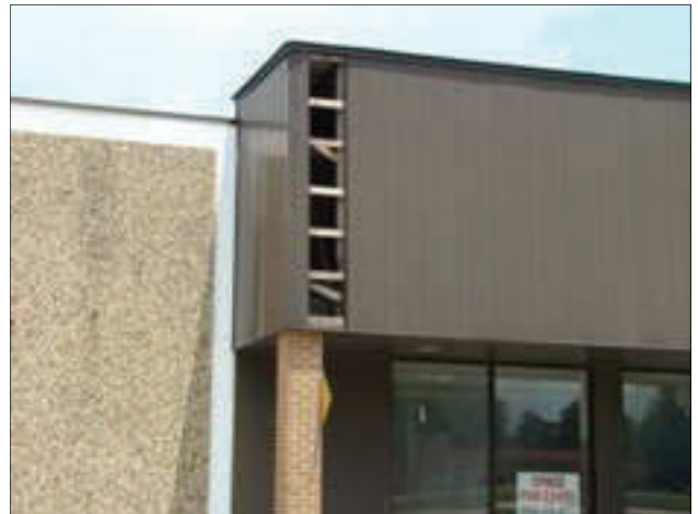
The vacant section the building housing Big Lots is missing sections of fascia exposing wood structural elements.
