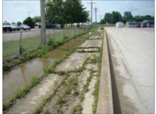
The drainage ditch running along the east side of the mall property is deteriorated and inadequate.
