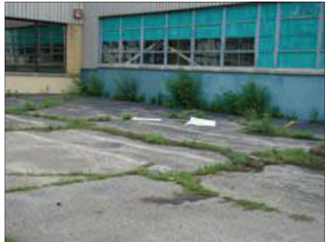
The front parking lot for Blaw Knox Ingersoll Rand is dilapidated. Note weed growth through cracks in the parking lot and along the foundation.
