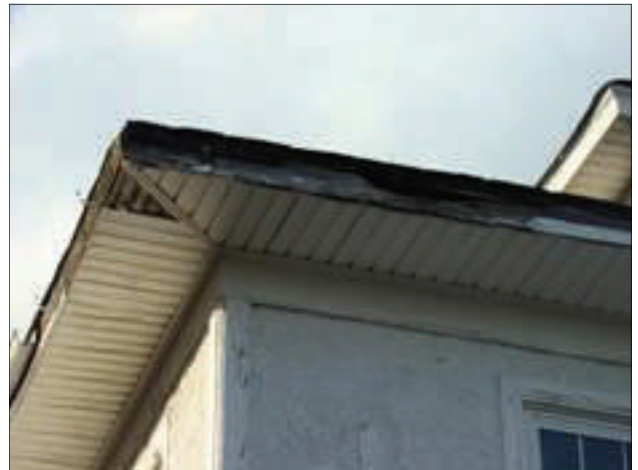
The fascia on the residential building shown at left is rotting.
