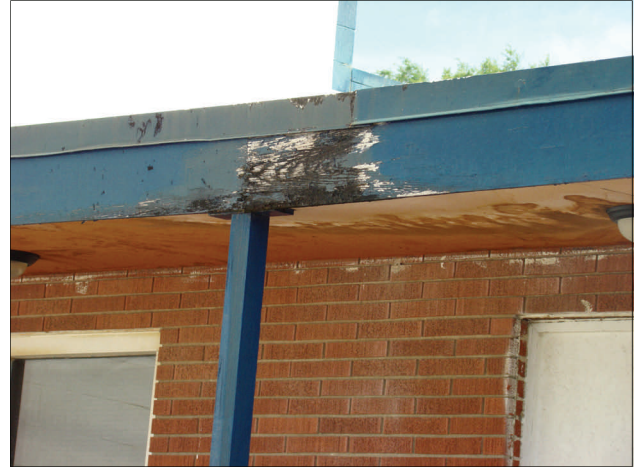
The front building on the Monitor parcel has severe water damage to the roof.
