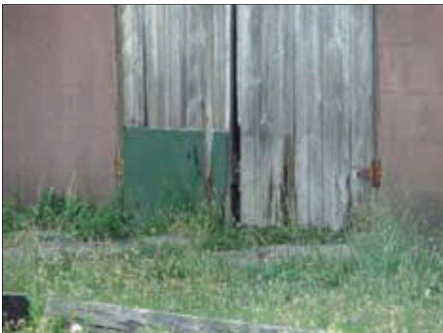
The door on the industrial property pictured above is rotting and has been patched with plywood.
