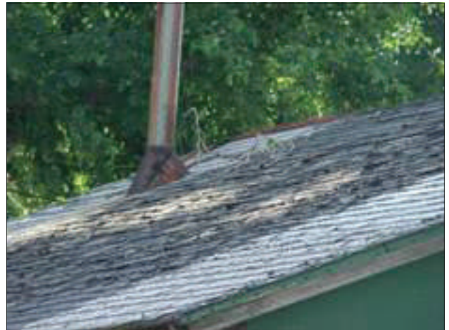
The roof of this industrial structure facing Division Avenue is in severe need of replacement.
