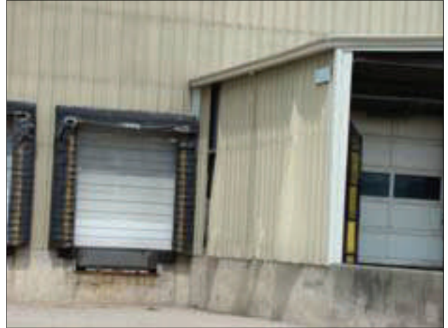
Sections of metal siding at the Alton facility are badly dented.
