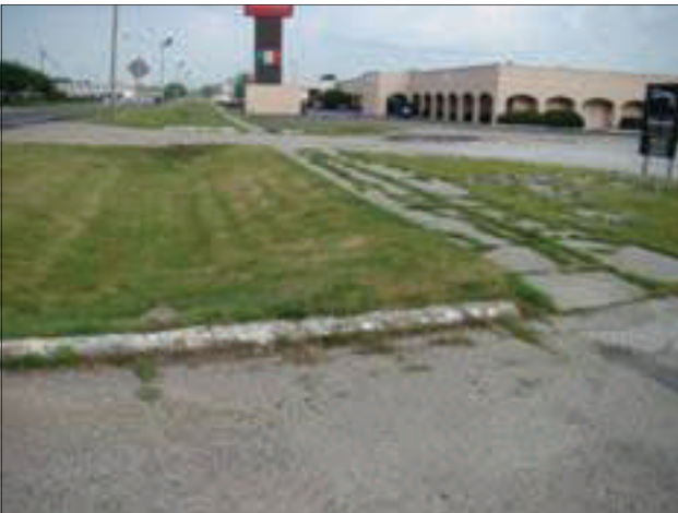
Many sections of sidewalk along Broadway are in severe need of repair or replacement.
