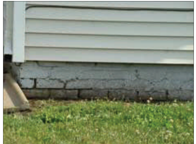
The brick foundation on this residential conversion is in need of tuck-pointing.
