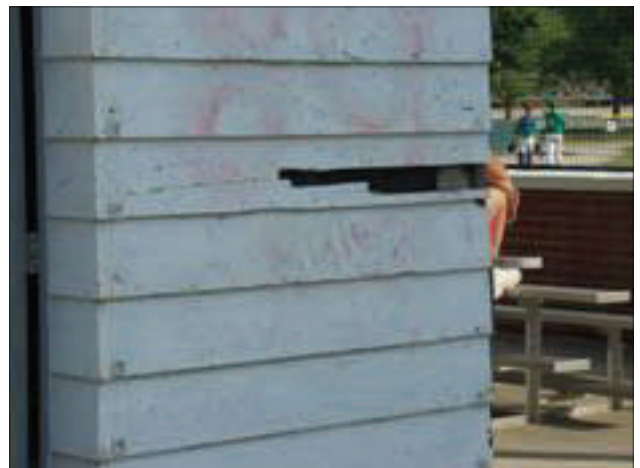
The siding of this structure in the park is rotting and sections are missing.
