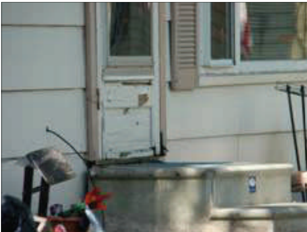
Rotting wood is observed on the front door of this single-family home on 1st Street.
