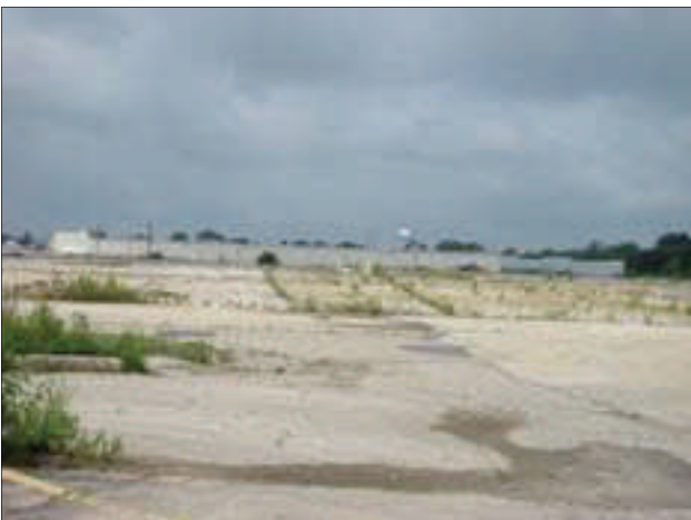
Rear parking lot for Blaw Knox Ingersoll Rand is also dilapidated.
