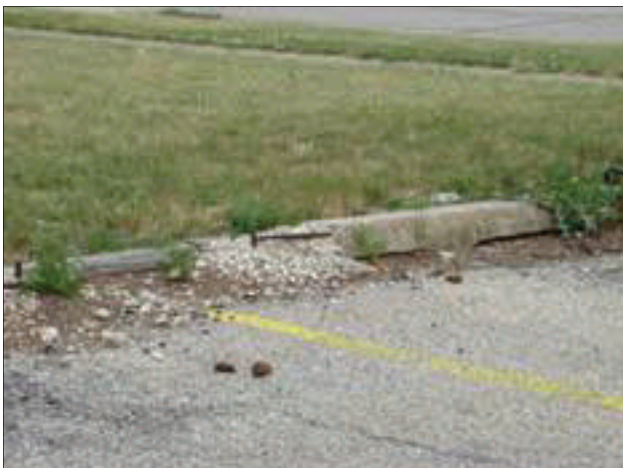
Concrete bumper blocks at the same medical office are disintegrating.
