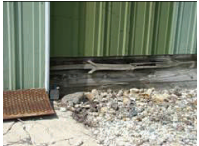
The wood foundation on the metal farm equipment building is rotting and splitting.
