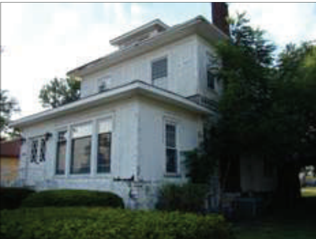
This brick on this single-family home has been covered with a stucco coating, which is now cracking and detaching from the masonry.
