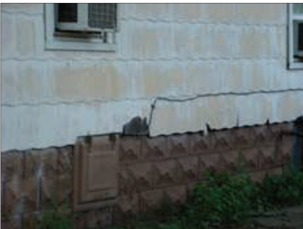
The siding on this residential building on Broadway is rotting and in need of replacement.
