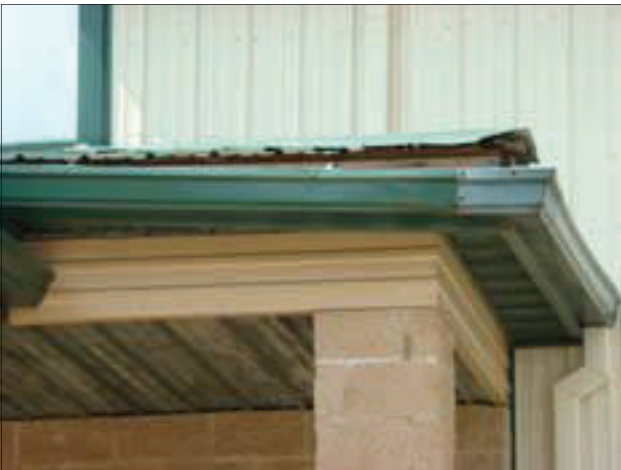
The gutter on the commercial building shown above is sagging and exposing the wood fascia board underneath.
