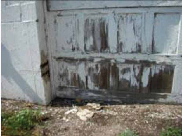
The garage door on this vacant industrial building is rotting.
