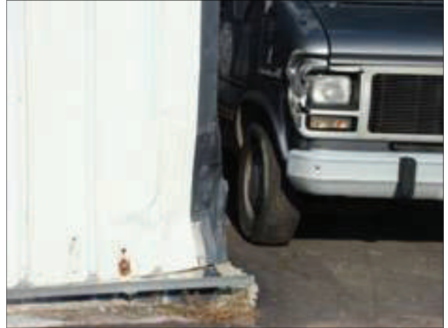
The siding on this steel shed is severely dented.
