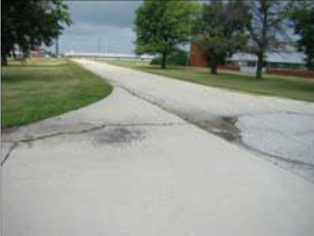
The access drive serving the Alton facility is cracked and crumbling.
