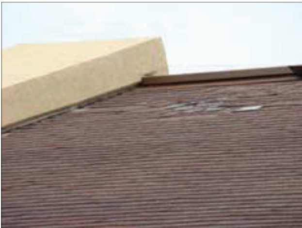
Shingles on the US Bank building are loose and a number of them have become completely dislodged.
